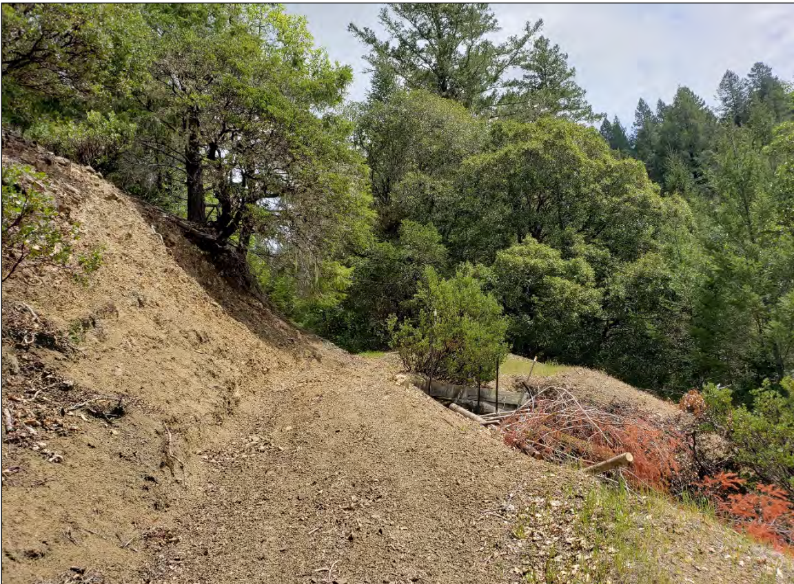
Photo 1: Poor road drainage placement (as seen on the Orange Trail) exacerbates this highly erosive landscape.
