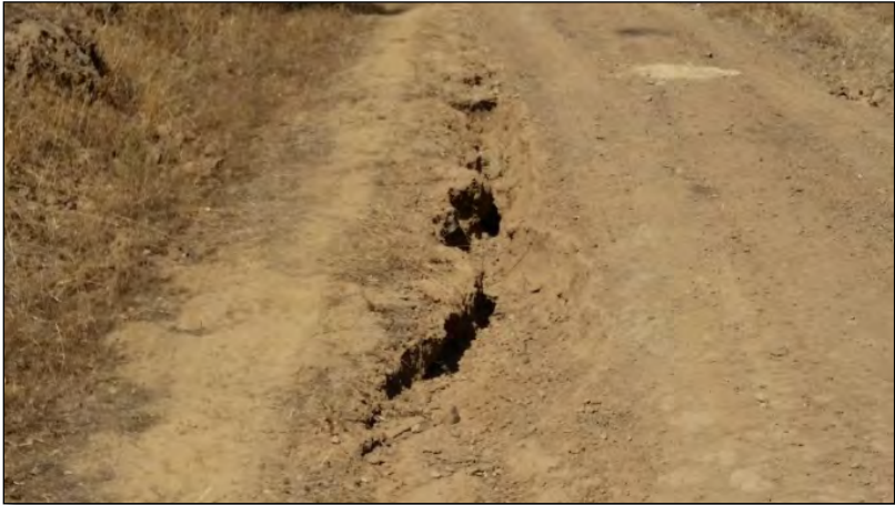
Photo 20: Evidence of rutting, reeling and erosion on the road surface is a sign of non-existent or improperly spaced erosion control features.
