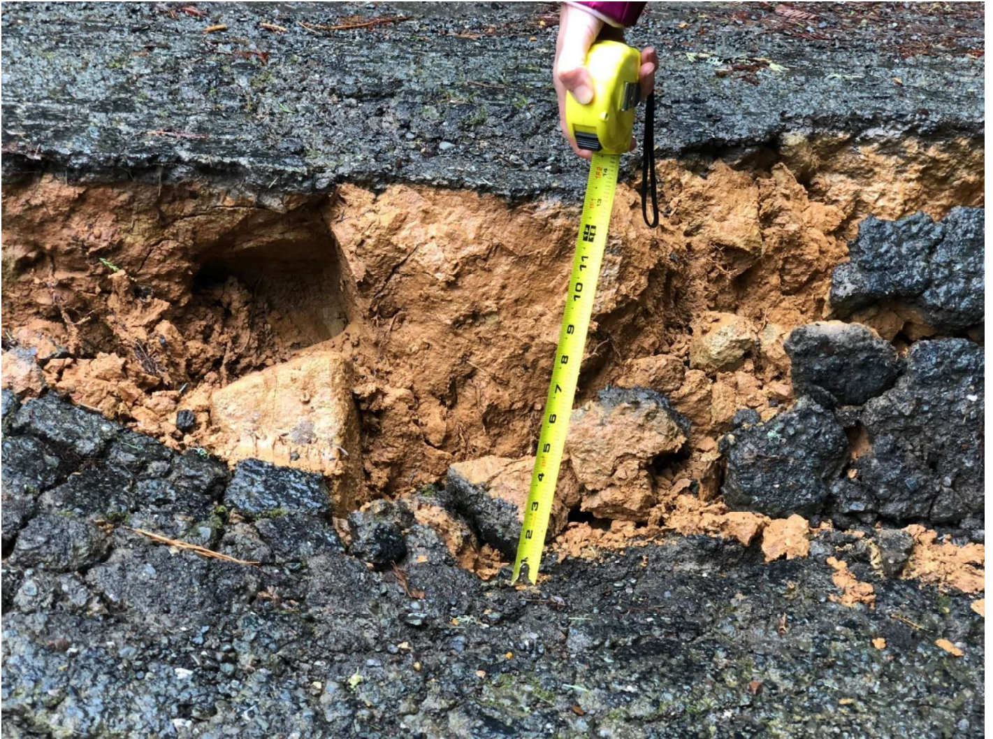
Photographed by Alina Haigler March 2019, post slumping. Soil displacement is approximately 1.2 vertical feet.
