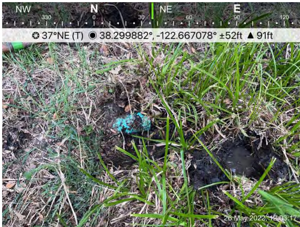
Photograph 4. View of what appears to be a broken pipe at first driveway on Adobe Road west of intersection. Broken pipe is presumed to be artificial source that likely resulted in Sample Point 2A meeting two of three wetland parameters.
