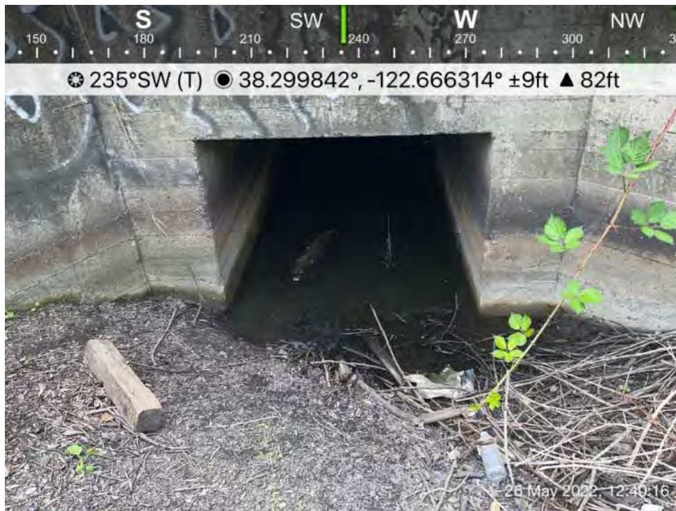
Photograph 6. View of concrete box culvert beneath northeast corner of intersection on (upstream side) of unnamed intermittent drainage.
