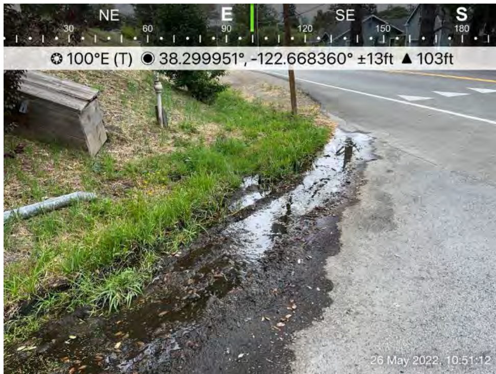
Photograph 2. View of likely broken pipe at entrance to Penngrove Elementary School just east and outside of Study Area on Adobe Road. Broken pipe is presumed to be artificial source of RD-01.
