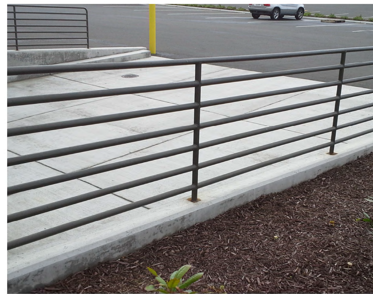
LOADING DOCK GUARDRAIL
