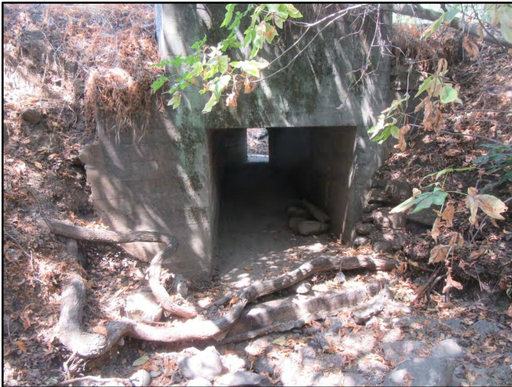
Culvert under a road in the northeast corner of the site, looking northwest; 07/03/18. Intermittent Stream IS-2 flows in to the site in this location.
