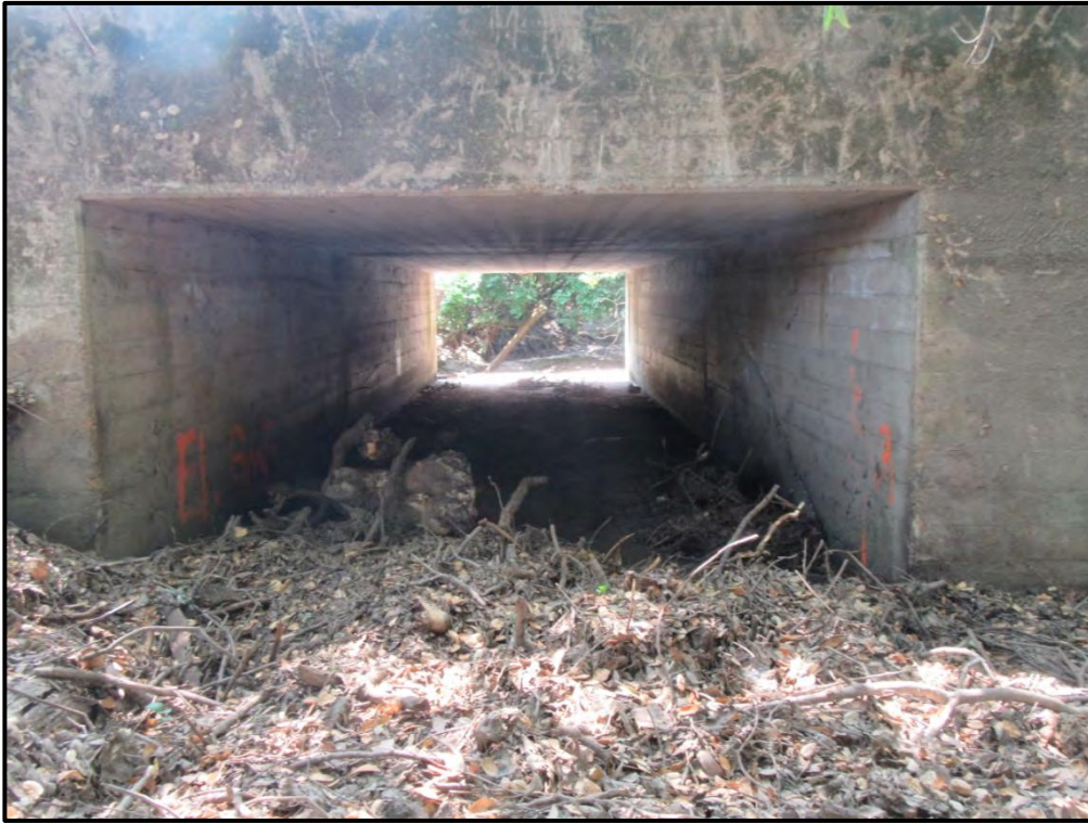
Culvert under Agua Caliente Road, looking southeast; 07/03/18. Intermittent Stream IS-1 continues southeast and drains in to Sonoma Creek.
