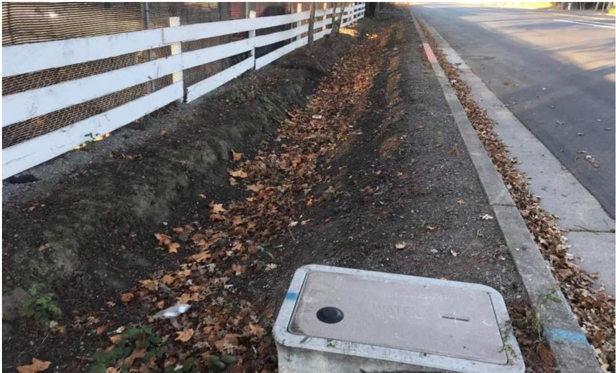
Photograph 16. View of drainage ditch on south side of Todd Road, from east end of easternmost segment, facing west.
