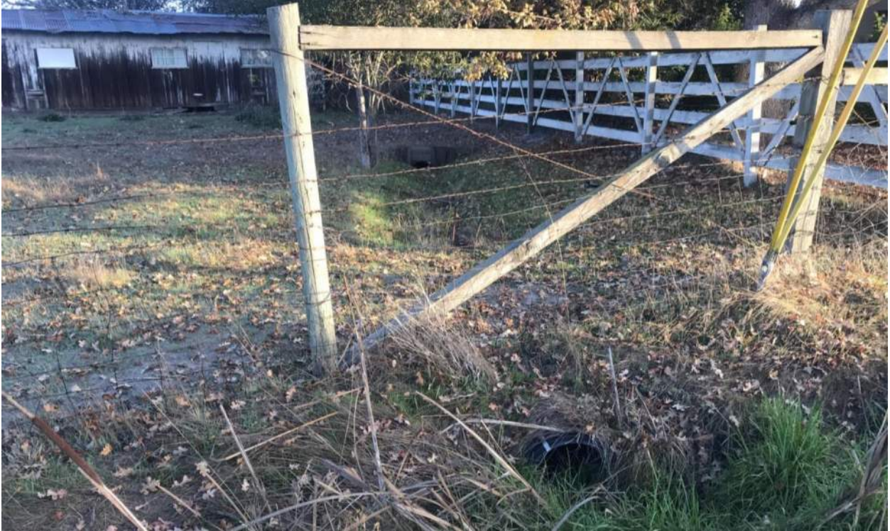
Photograph 9. View of fork in drainage ditch on north side of Todd Road where it turns to drain into ruderal area on property to north, facing north.
