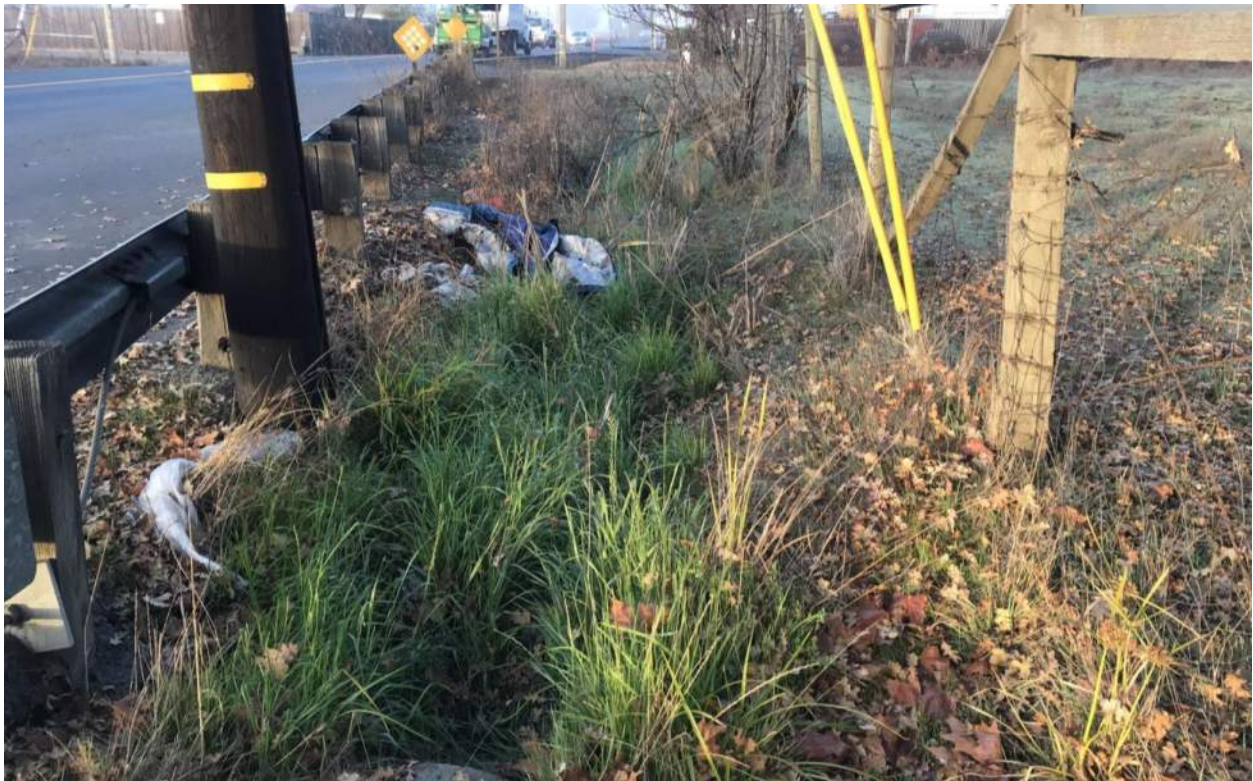
Photograph 8. Eastern end of drainage ditch on north side of Todd Road, facing west. Concrete inlet to storm drain system visible in foreground.
