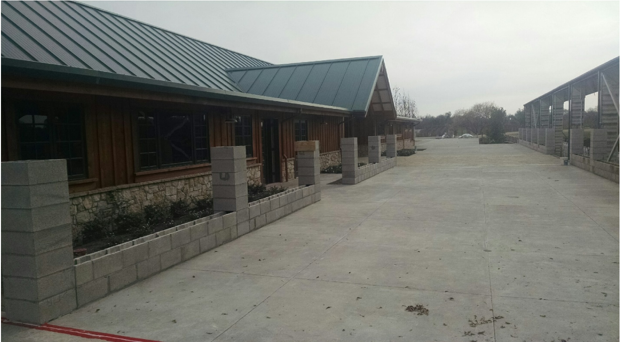
View of existing “agricultural barn” that is undergoing renovation for the proposed winery use
