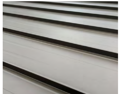
ROOF 01: METAL ROOFING > Standing seam metal roofing color "slate grey" LRV 12 . See spec sheet.
